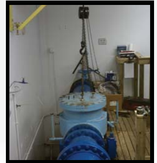
16" GA Valve in Glenwood, IL
